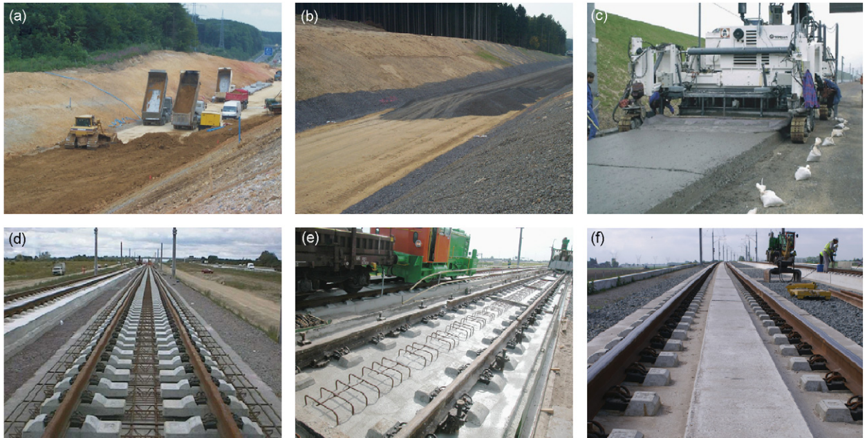
Fig. 1. Different stages of installation of a slab track railway system: (a, b) soil improvement, (c) automated installation of HSL-layer (see Fig. 2; class B5, without reinforcement), (d) installation of duoblock sleepers and central reinforcement, (e) in situ casting of the concrete track, (f) finished continuous concrete railway track.
